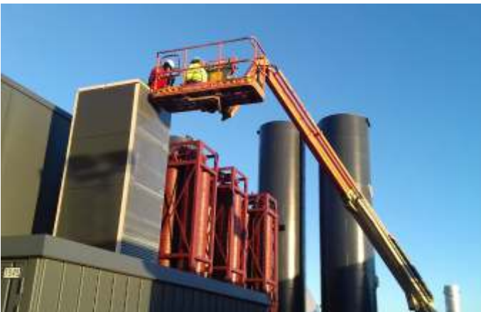
Site installation of HEX batteries
